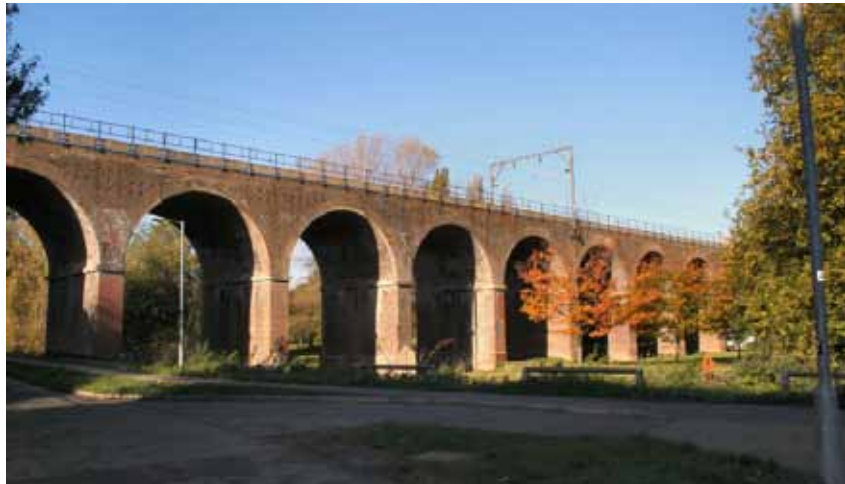
A section of the Chelmsford viaduct in Central Park © Stuart Axe via Wikimedia Commons
