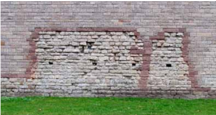
Sections of Roman wall at Cardiff Castle Rory Walsh © RGS-IBG Discovering Britain
