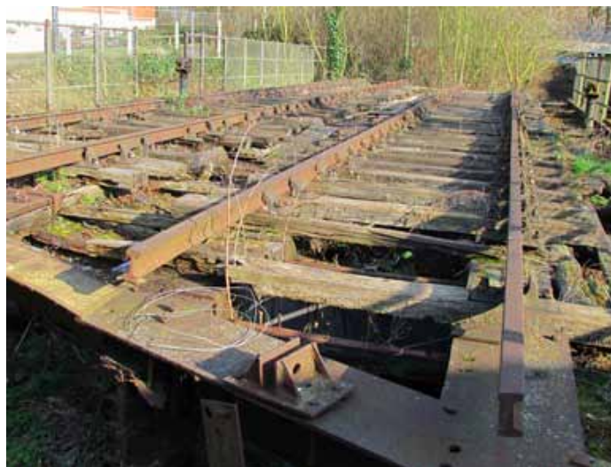
The swing bridge is currently awaiting restoration Rory Walsh © RGS-IBG Discovering Britain
