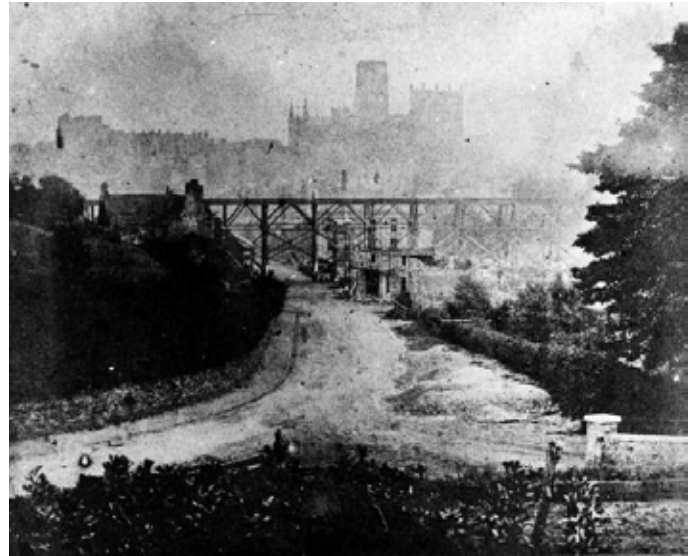
Construction of Durham railway viaduct (c.1855) Reproduced by permission of Durham County Record Office (Ref: D/CI 27/277/296)
