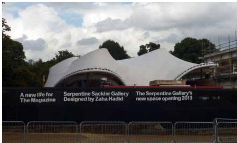
The Serpentine Sackler Gallery under construction © Julian Osley, Geograph (Creative Commons License)
